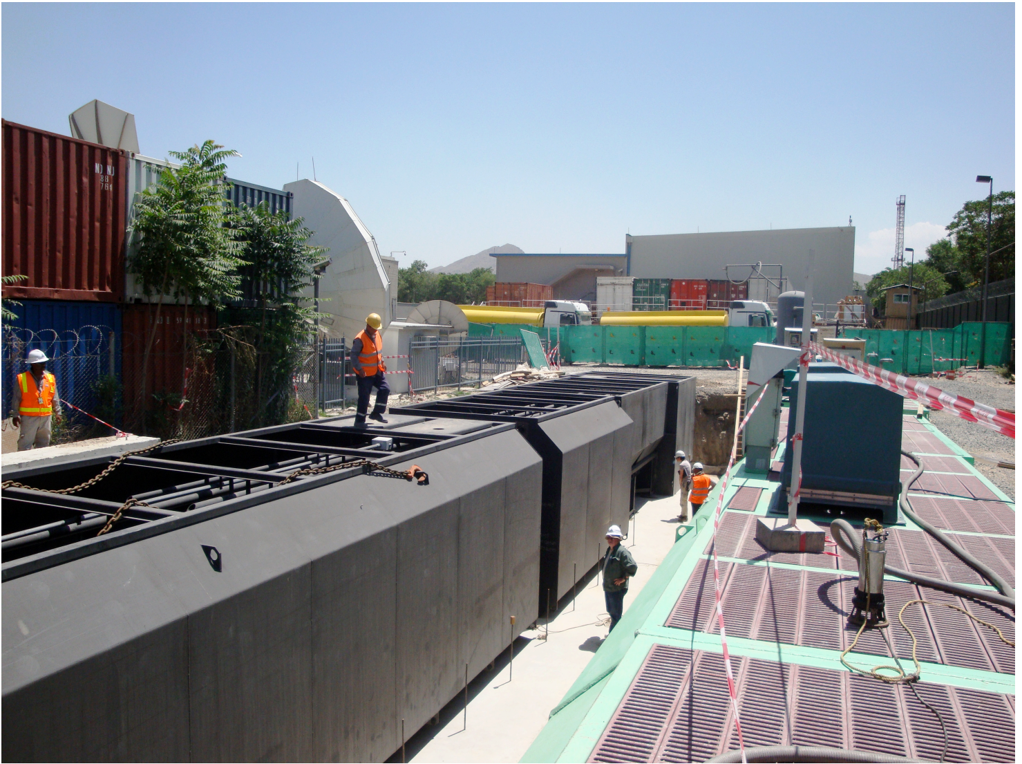
US Embassy Kabul, Afghanistan Dual 40,000 GPD Prefabricated steel secondary & dual media tertiary filters.
