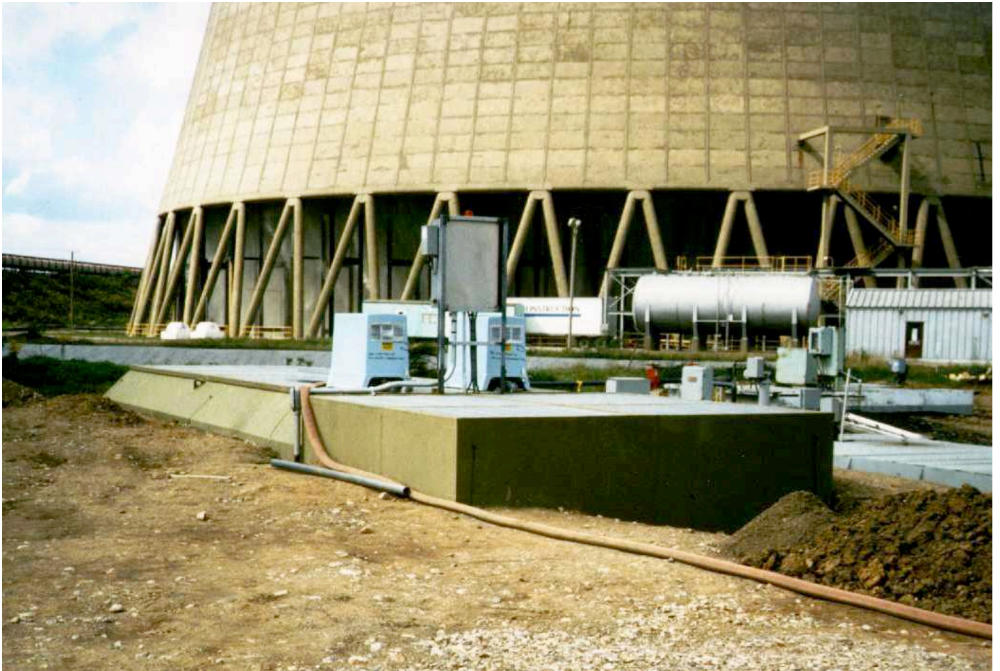
Ohio River Power Station, 10,000 GPD Prefabricated steel secondary treatment system.
