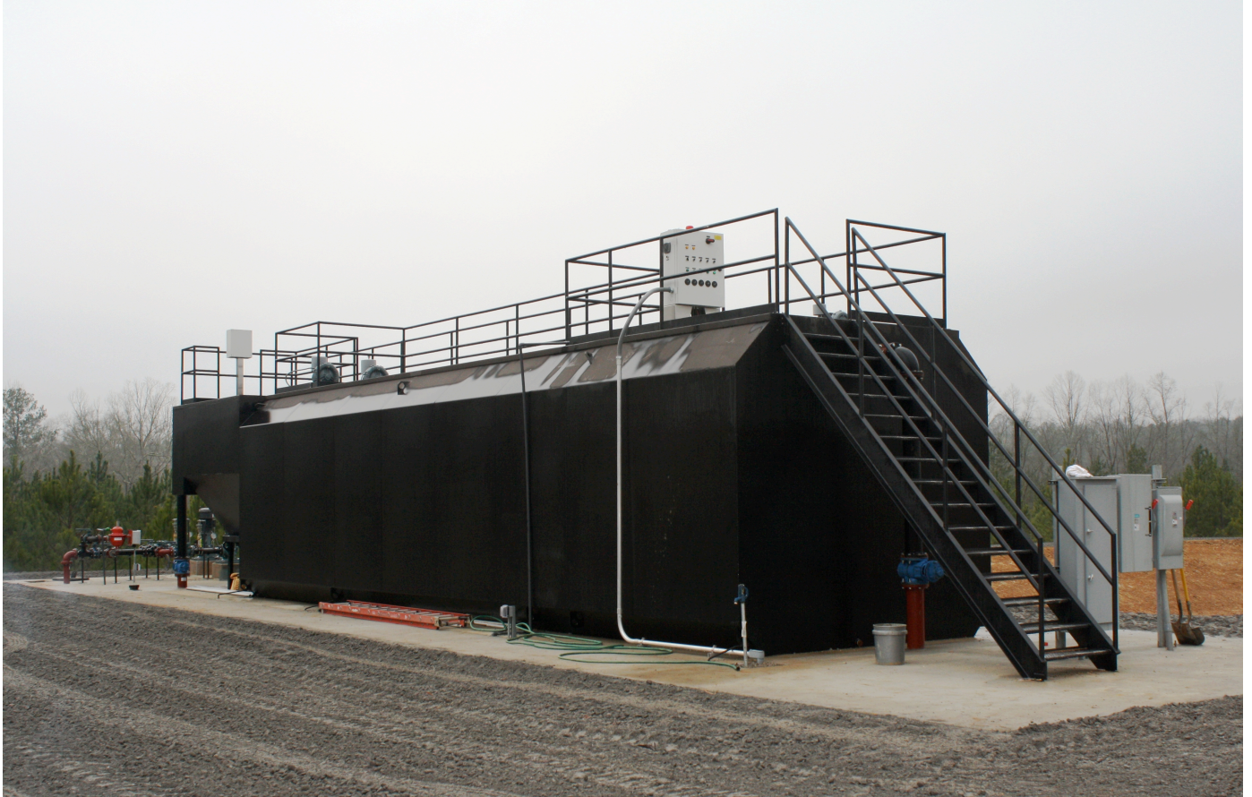
Holliday Inn, Guin, Alabama. 25,000 GPD Prefabricated steel secondary treatment system, with spray field irrigation system.
